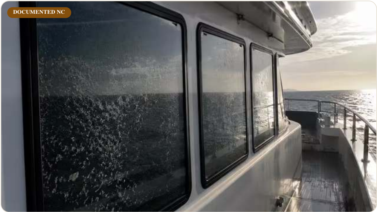
Wide shot of the port deck against the light, crystallised salt visible on the 3 glass panels.
